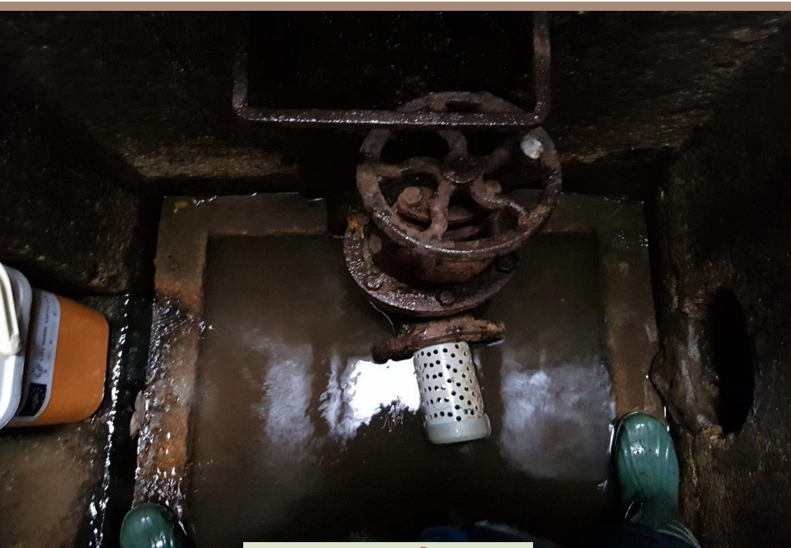
Improperly maintained Model 2 spring box.
