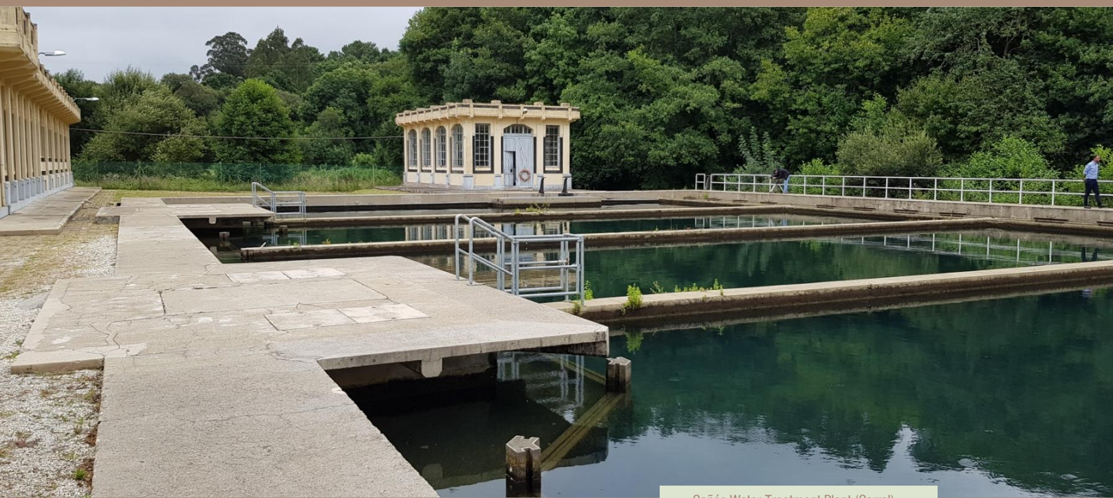
Cañas Water Treatment Plant (Carral)
